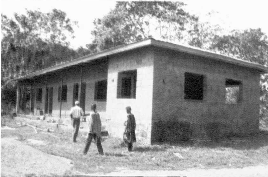
a block of 3 classrooms under construction at Igboodu- a product of Manos unidas intervention
